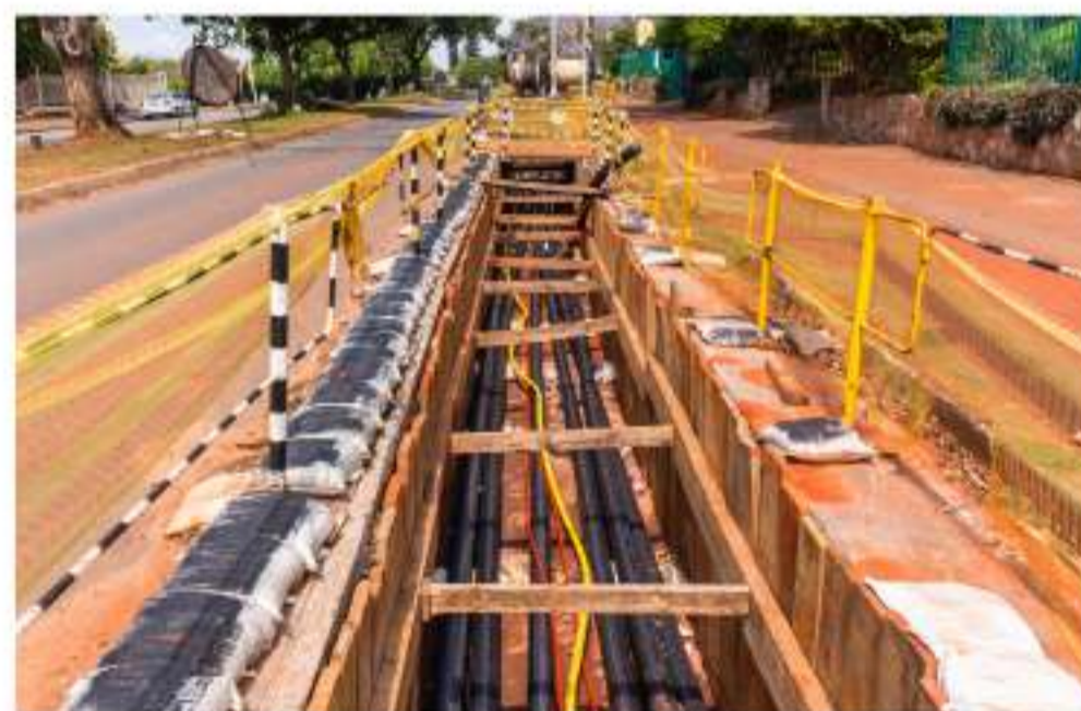
Underground electricity and infrastructure for safety and aesthetics.
